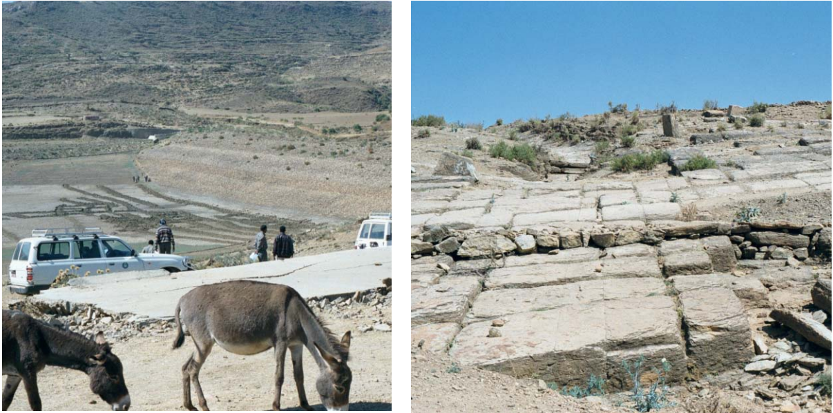
Figure 6. (a) Dam in northern Ethiopia that lost water at a high rate because of leakage through the cavernous limestones that underlie the reservoir. (b) Detail of the jointed, cavernous limestones that form the substrate of the dam.
